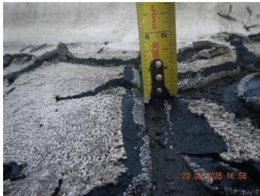
Photo 5 – Cracked roof coating material. Cap sheet also appears to be damaged.
